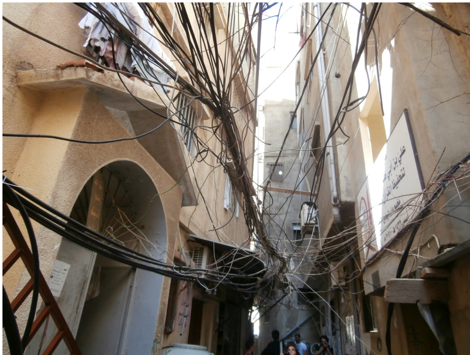
In spiraling alleys of squalid dwellings, a tangled maze of live power lines supplies electricity (2009). Photo courtesy of the author.
